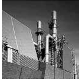
Fig 4. UCLA Chiller Plant & Cogeneration Facility
